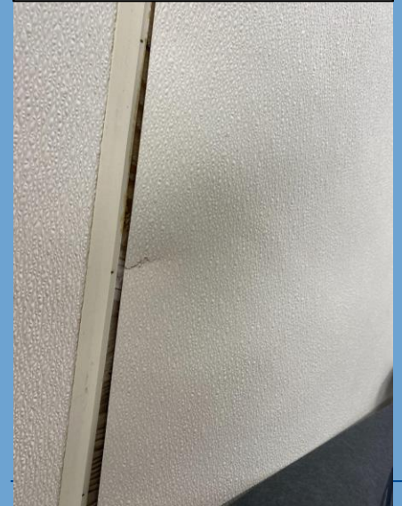
Meat Dept. wall is warped due to black mold behind the panel
